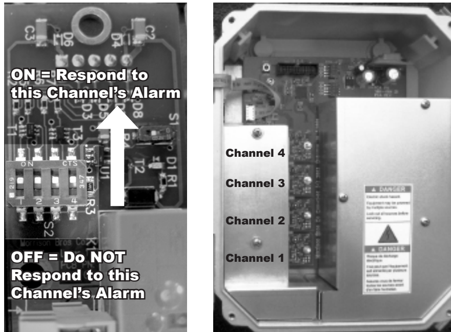
Figure 8 - Output Module Alarm Channel Configuration
